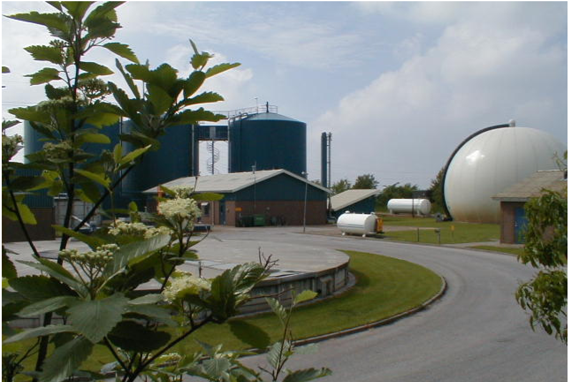
Ribe Biogas; 15 years of production, 18.000 m 3 biogas/day. .Source J. B. Holm-Nielsen, Bioenergy Dept., SDU, Denmark.
